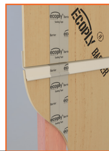
Corner Profile Sealing tape applied to Ecoply above and placed over 'Z' flashing at corner junction OR Ecoply Barrier 150 mm Frame Sealing Tape
